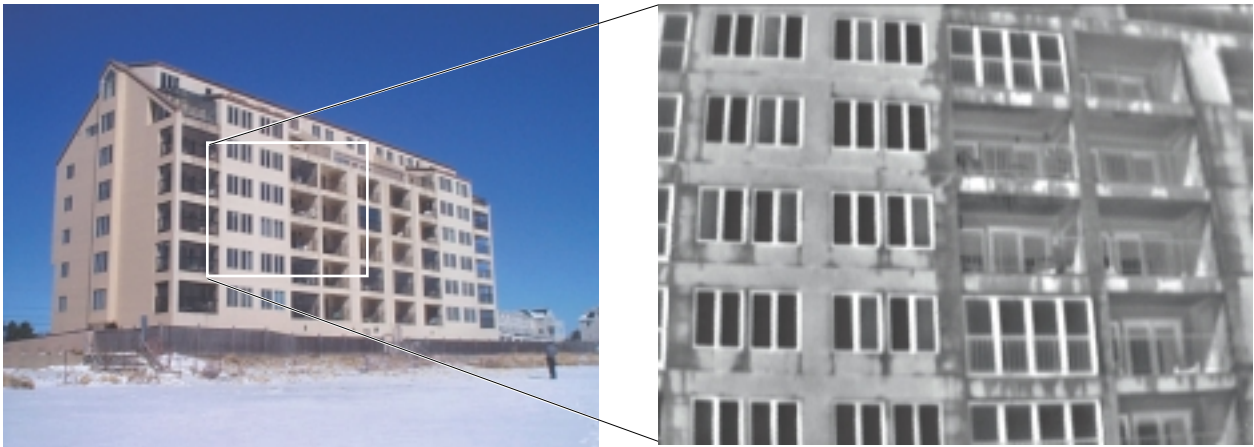
Figure 10. Rainwater entering through cracks in EIFS can lead to mold growth. IR images show moisture accumulation here.
