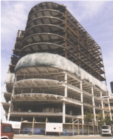
Figure 5. In high-rise construction, water from upper stories can wet lower finished floors.
